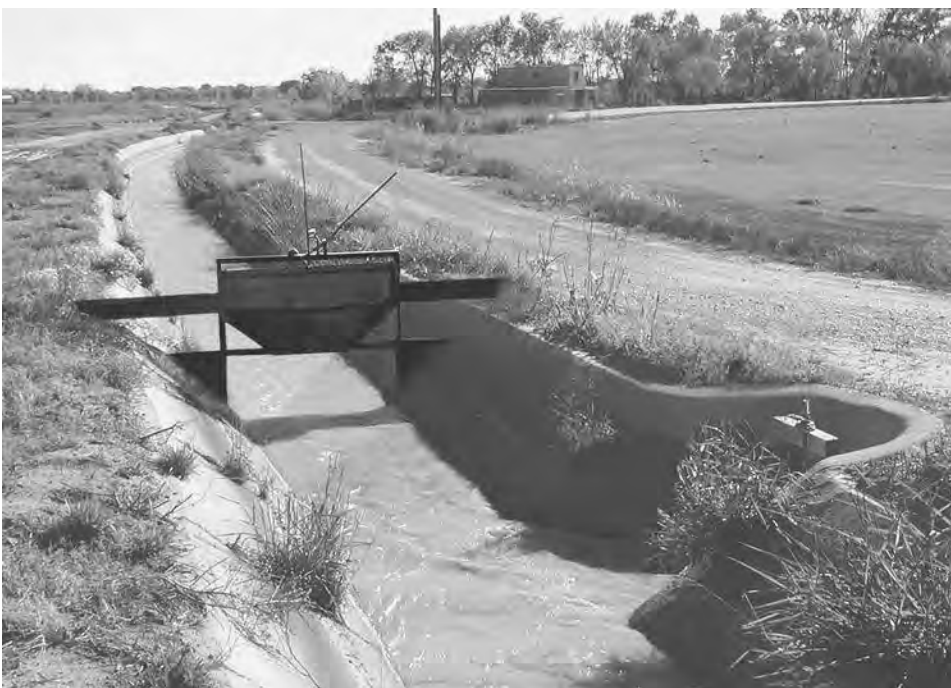
The metal structure on the left is a check. When it is closed the water in the high-line canal or lateral builds up to a level that will flow through the turnout, shown at lower right, into a farm field or smaller ditch.
